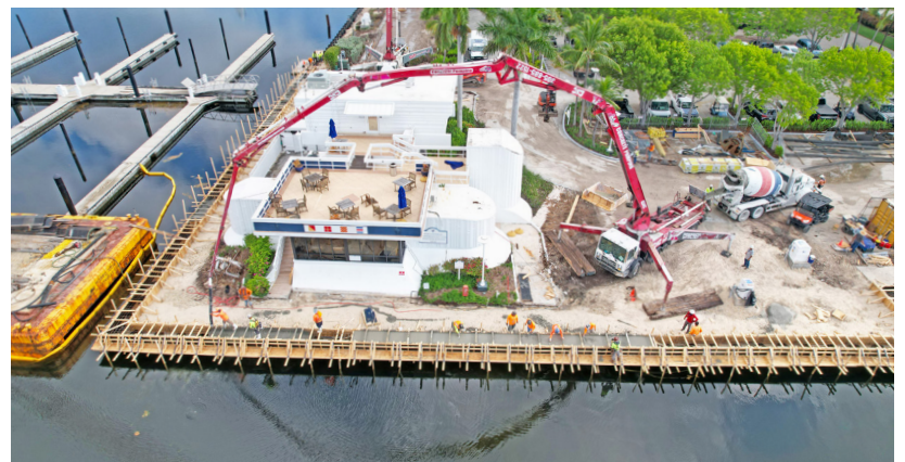
Fuel Dock and D Dock concrete cap pour in progress, photographed June 9.
