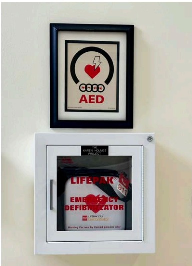
Sixty-five of these lifesaving AEDs are located throughout The Reef.
